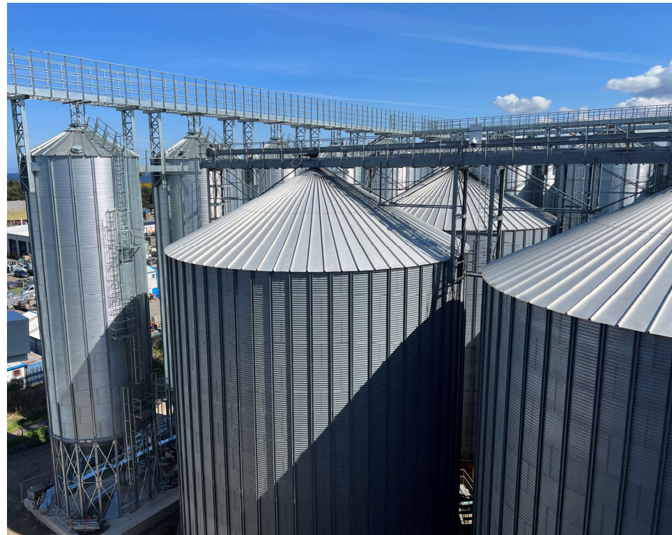
New malt storage bins as part of additional malt storage, cleaning and out loading facility
